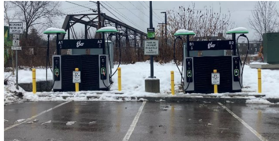
Example 2: EVSE in a public parking lot owned by a public utility open to anyone who would like to use it and charging the general public by kWh and time.
