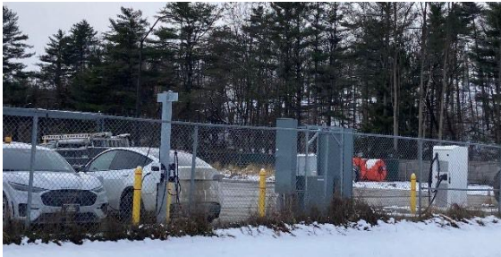
Example 1: EVSE behind a fence owned by a public utility for their exclusive use.
